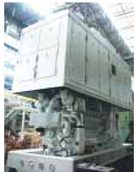
■ Fig. 7 – Diesel generator set with double resilient mounting and acoustic enclosure.
